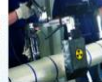
Infrastructure Health (SHM)
